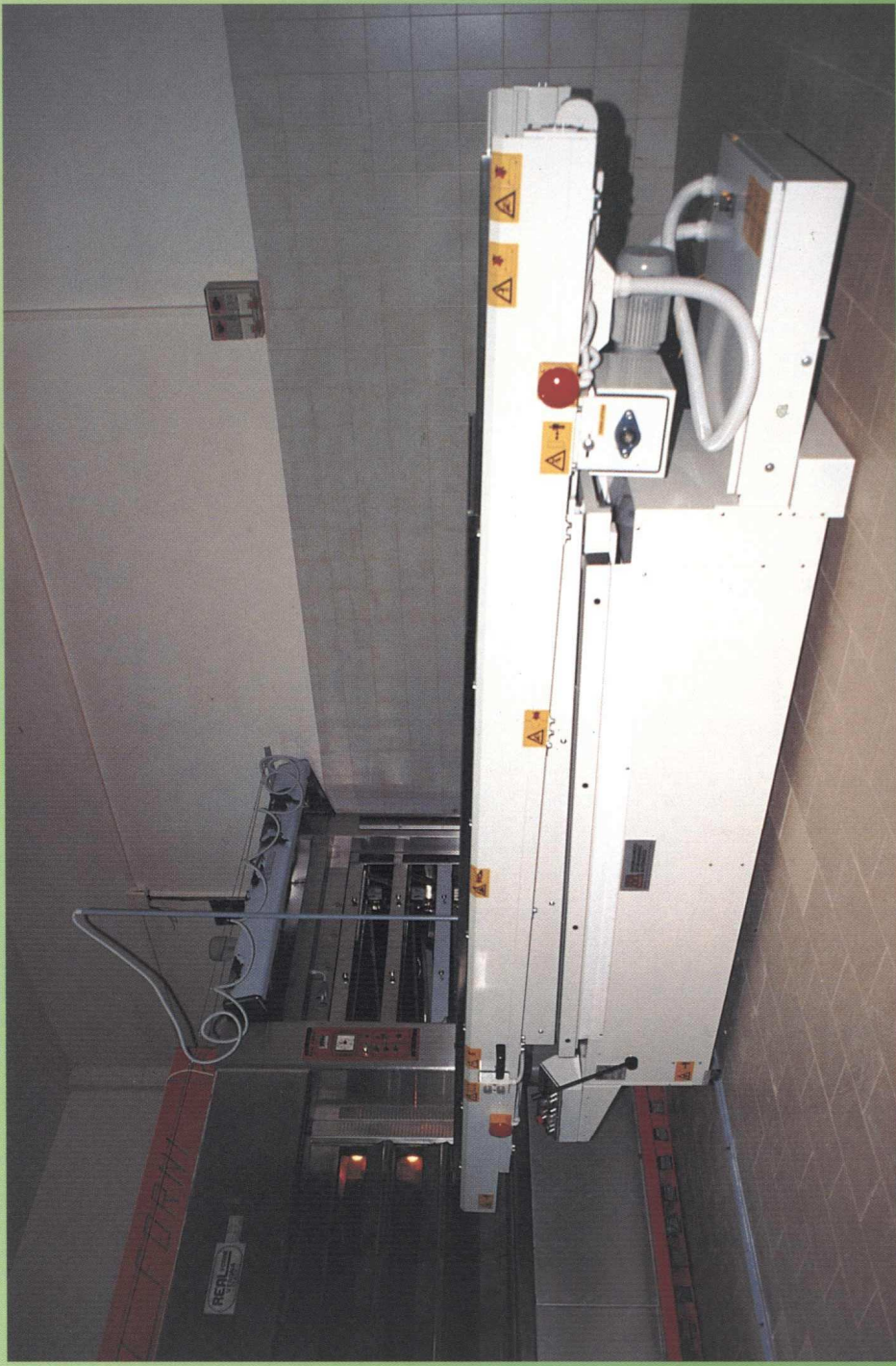
Impianto con pala "PF" Plant with "PF" baker's shovel
